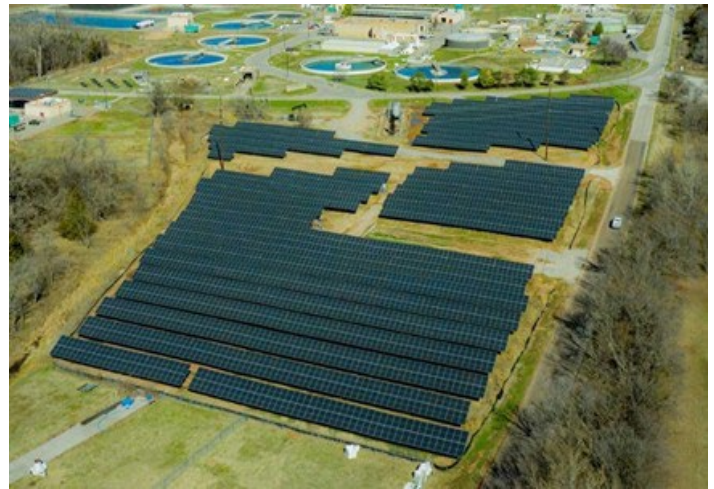
Figure 9: Solar Array in Norman 17
